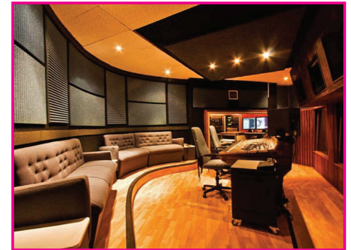
Acoustic panels and Ceiling Clouds
